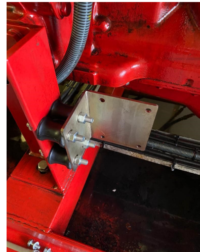
Installed Anti-Vibration Kit (PVAC)
